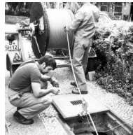
First German telecom cable
