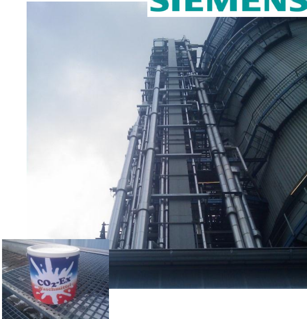
Pilot scale test of CO 2 capture with Amino-Acid Salts in PP Staudinger (Siemens)
