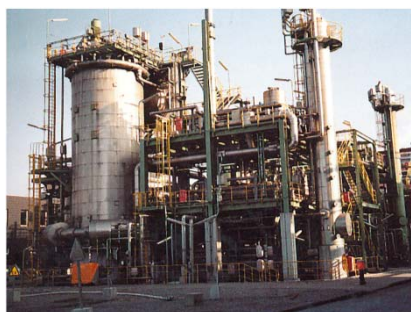
OXEA plant in Oberhausen
